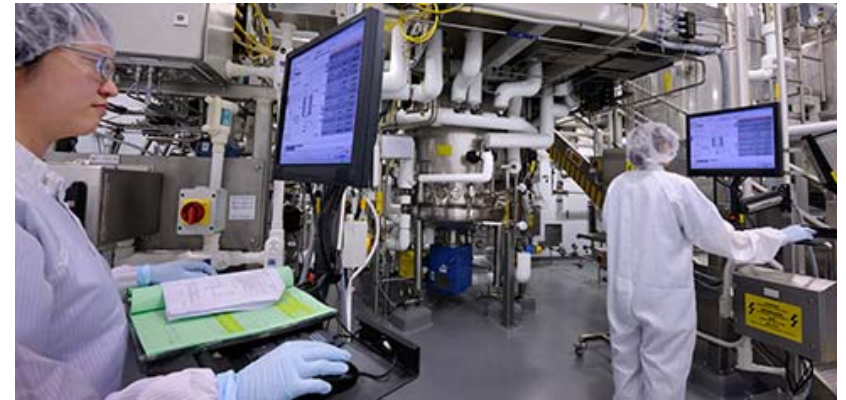
Inside a TBP facility, source: www.jtc.gov.sg
