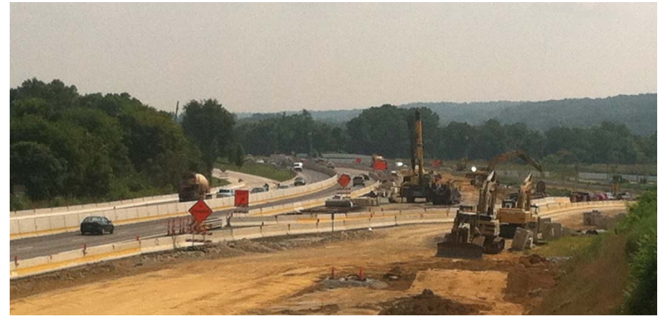
A recent view of the Route 202 widening project from the Route 29 overpass in Malvern
